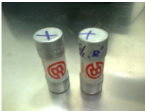
The fuse is burnt 4 times one year
